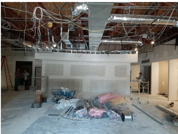
The contractor for the Evergreen remodel finished the drywall and began painting this month. The service desk area is shown in the photo.
